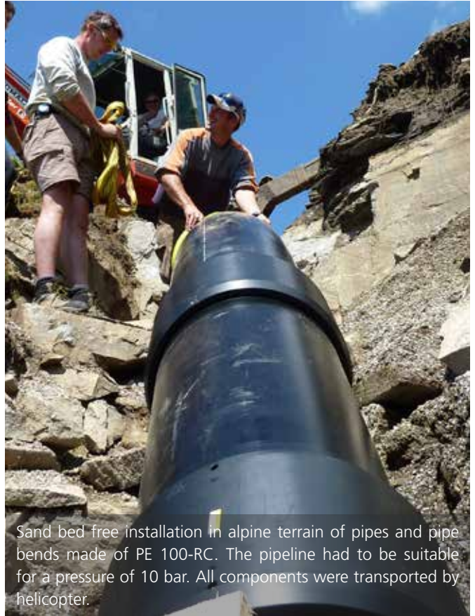
AGRU Kunststofftechnik supplied several hundred meters of PE 100-RC pipes in outside diameters between OD 560 mm and OD 710 mm for a new district cooling center in Vienna.
